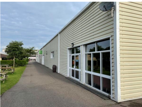
4.5 SE corner of premises which shall receive adaptation to accommodate retail offer
